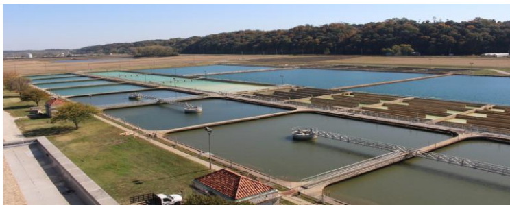
Howard Bend Plant
